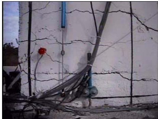
Fig. 9 Extent of flexure-shear cracking at the bottom corner of the first story of the web wall during EQ4 (at instant of time near maximum base rotation)
